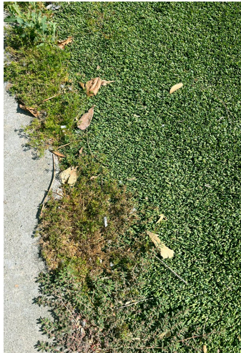
Weeds can grow in artificial turf if not maintained and controlled properly
